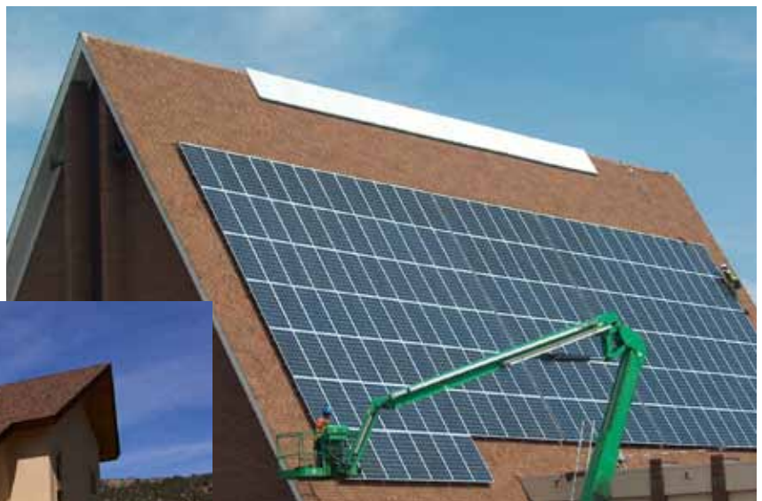
Mountain View UMC's Solar Panels consecrated May 1, 2011.
